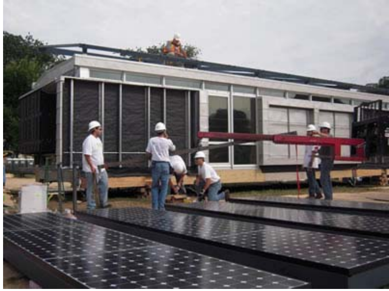
Crew members from the University of Kentucky prepare to install their house's solar electric panels. Photo by Ismael Martinez, courtesy of U.S. Department of Energy Solar Decathlon.
